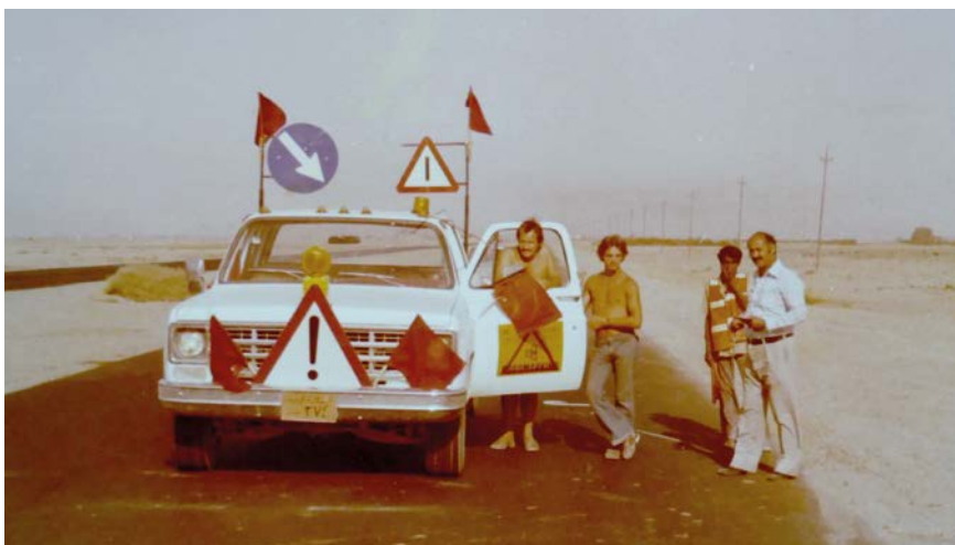
A "safety car" for the safety of the striping crew during their hard work
