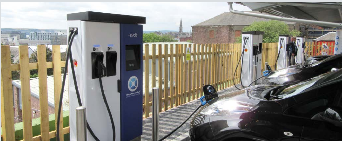
Almost 7000 e-vehicle charge points from SWARCO are in operation in the UK
